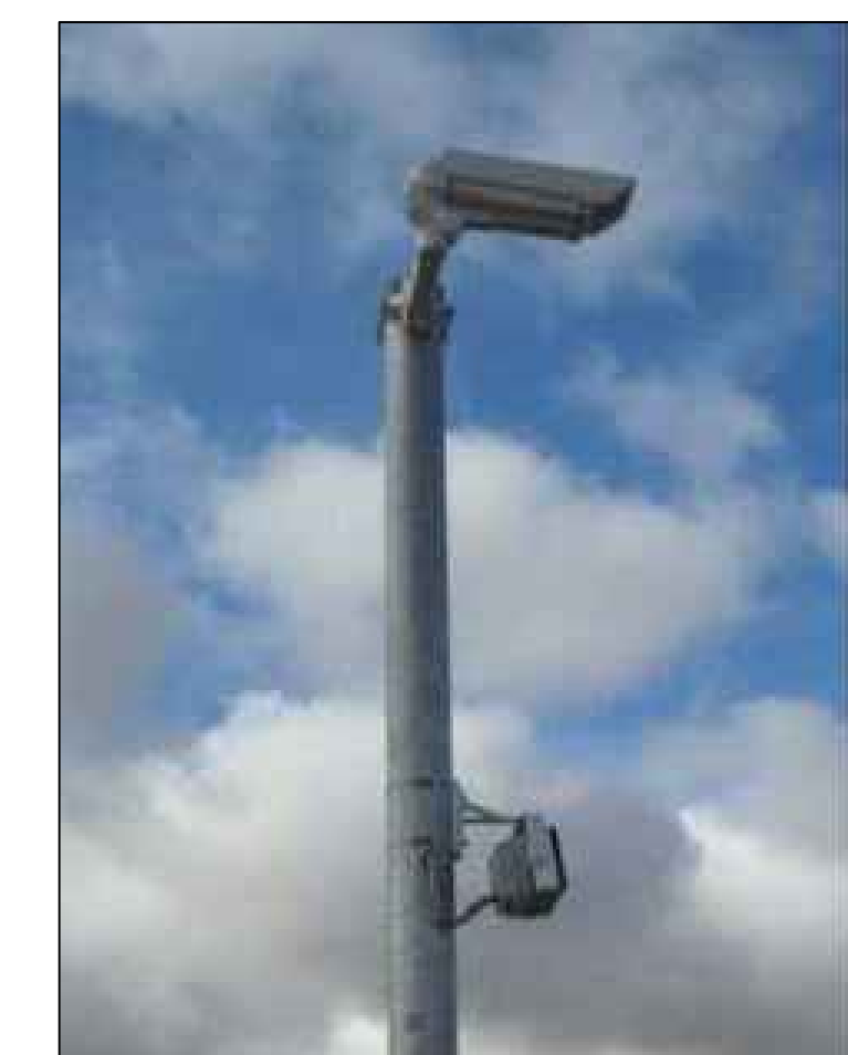
TYPICAL IMAGE OF CCTV CAMERA
